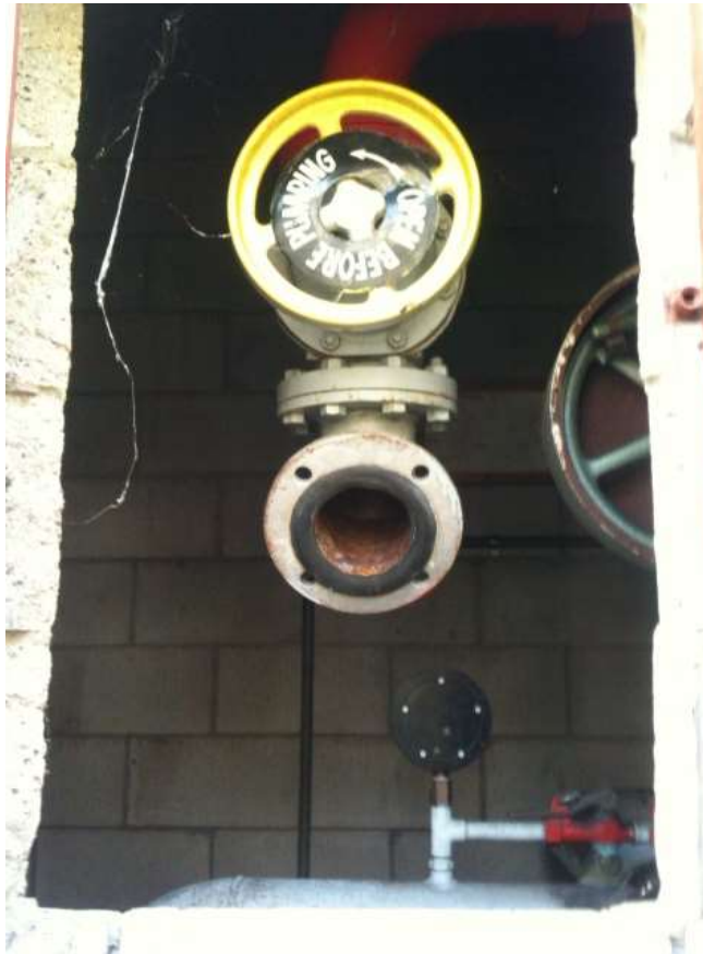
Missing inlet manifold
