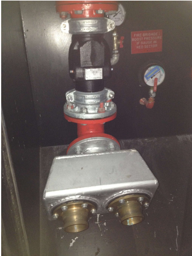
Typical inlet manifold
