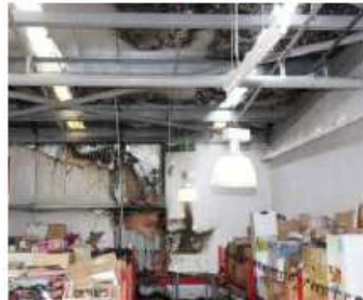
Above: the rapid fire spread was promoted by flammable surface linings
